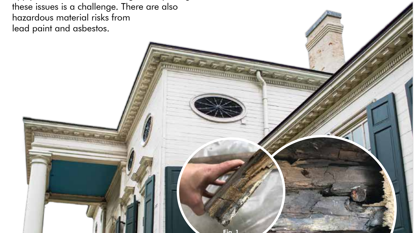
Fig. 1 | Tests were completed throughout 21 different areas of the historic home in spring 2019. This photo of a piece of siding from the historic house shows the severe water penetration (left side of the board in photo) representative of the conditions discovered in some of the lower portions of the walls.
